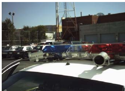
Fig. 3. Example of Auto-Detector installation for the Italian Carabinieri-Arm, the Italian Road Police, and USA State Highway Patrol forces
